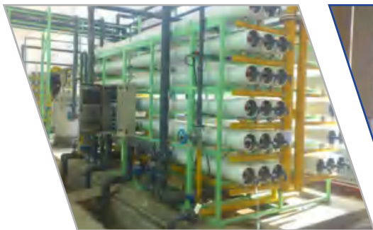
Gansu chemical plant water process engineering. May 2014
